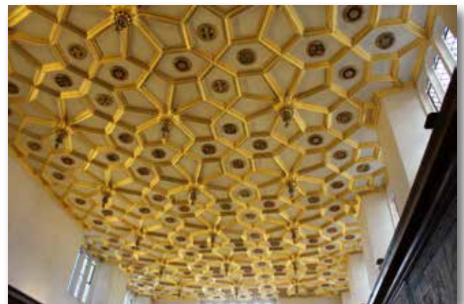
Photo of the ceiling of the waiting hall at Hampton Court © Tim Ridgway 2012
